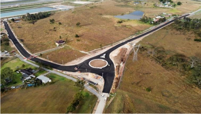
Progress of the new round-a-bout at the Adams Road and Anton Road intersection, taken August 2022
