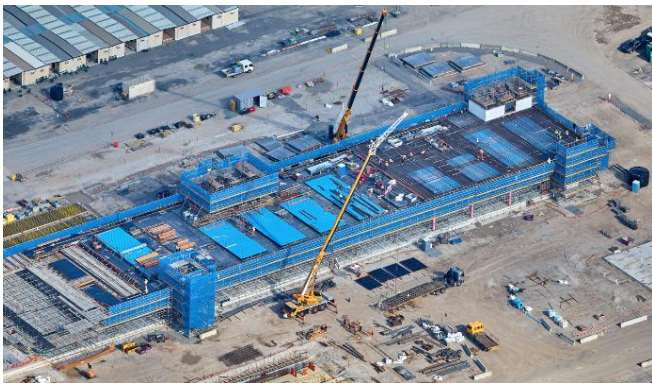
Aerial photo of the western pier on the terminal site, taken August 2022
